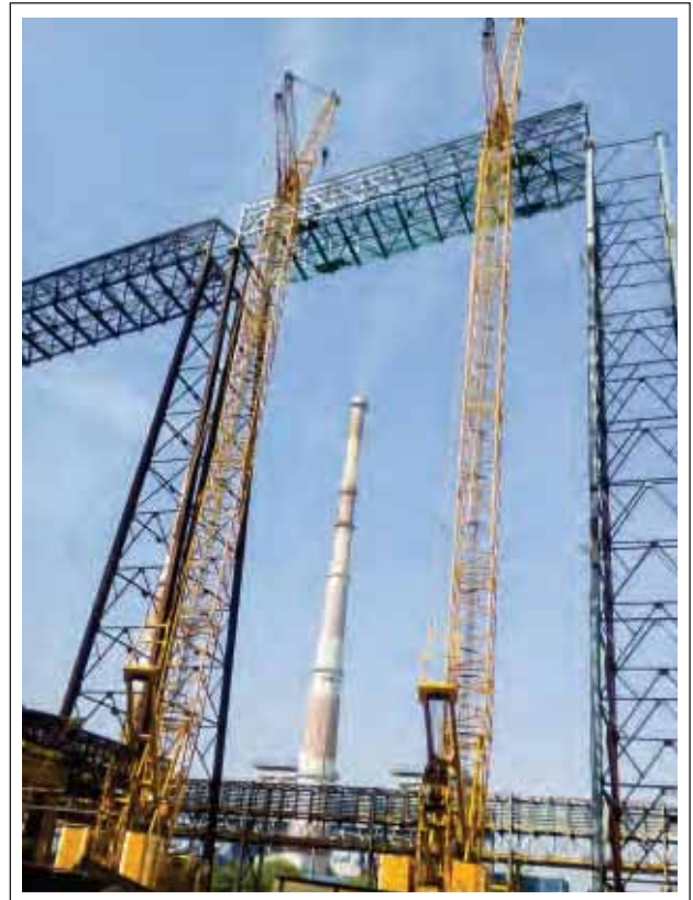
SANY SCC 2500C Crawler Cranes (Capacity 250MT) two nos. erecting 52MT in tandem with luffing configuration for Lanco Infratech Ltd, Korba, Chhattisgarh
