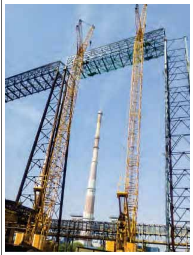
SANY SCC 2500C Crawler Cranes (Capacity 250MT) two nos. erecting 52MT in tandem with luffing configuration for Lanco Infratech Ltd, Korba, Chhattisgarh
