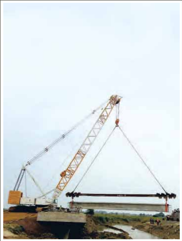
DEMAG CC 2400 (Capacity 450 MT) Crawler Crane, main boom 36M erecting Bridge Girder 80 MT at Afcons Infrastructure Limited site at Etawah, Uttar Pradesh
