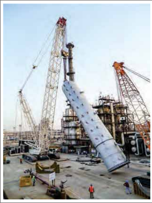
TERREX DEMAG CC 2400-1 (Capacity 400MT) Crawler mounted lattice boom Crane in SSL- 48Mtrs configuration erecting column of 210MT at KKSEPL, IOCL VADODRA
