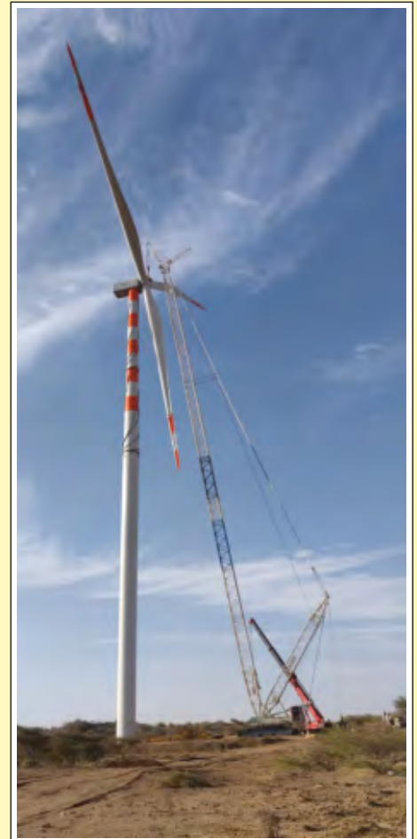
▶ Terex-Demag CC 2800/1 (SSL LSL + LF2 SGL_S7 (114 m + 12 m, 600 MT crawler crane) working in Gadhsisa Wind Farm, Gujarat.
