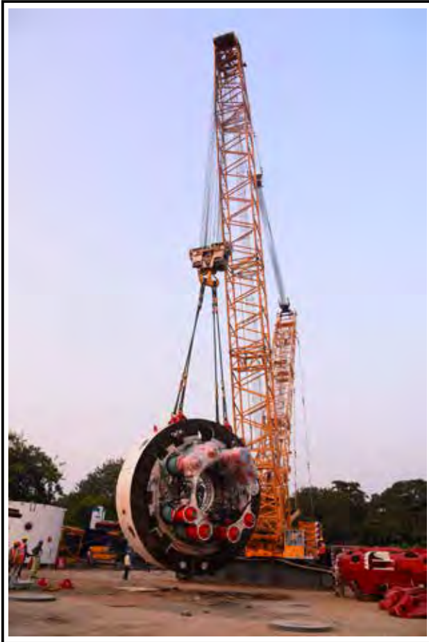
Liebherr LR 1400/2 SDB 35 m handling TBM components with a maximum load of 180 MT at MMRC, Mumbai.
