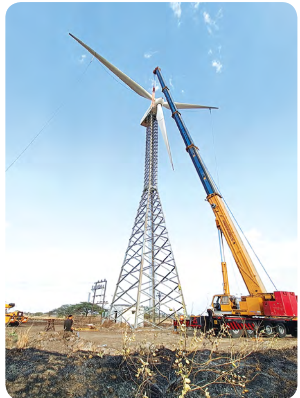
Groove GMK6300 (300 MT Crane) deployed at windfarm for operation & maintenance job handling 35 MT Nacelle at the hub height of 48m Nagar District of Maharashtra
