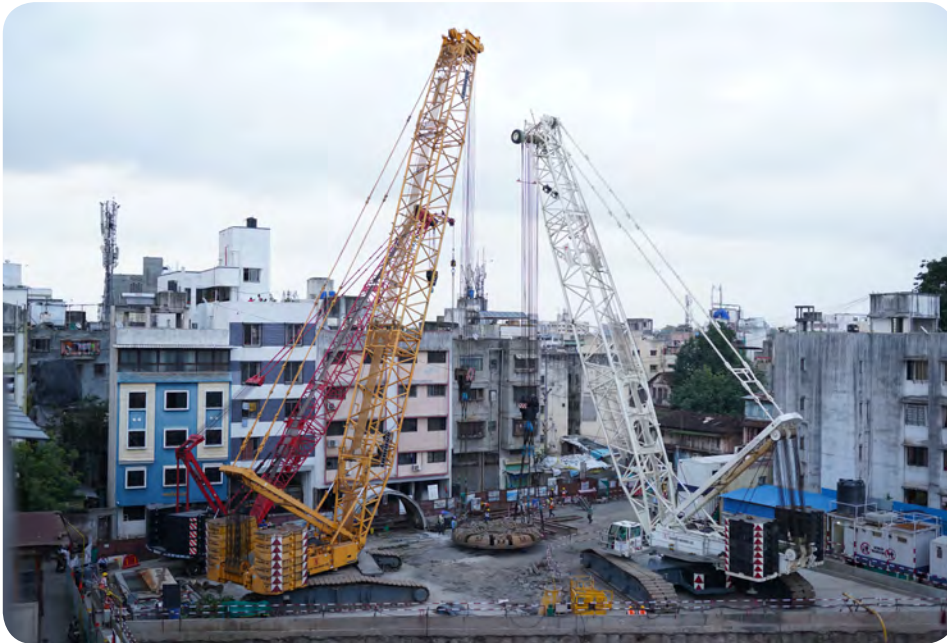
Terex CC2800-1 (600 MT lifting Capacity) along with Liebherr LR1400-2 deployed in Metro Railway Project, handling Tunnel Boring Machine (TBM) weighing 145 MT at one of the busy locality in Pune, Maharashtra
